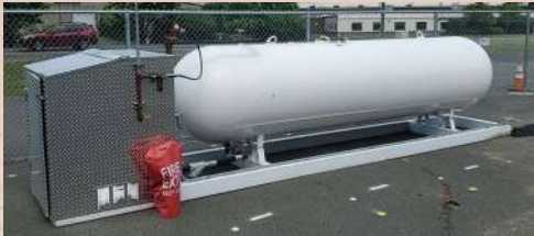
New Bulk Propane Tank Filling Station
