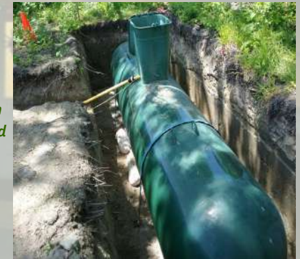
1000 Gallon Underground Tank
