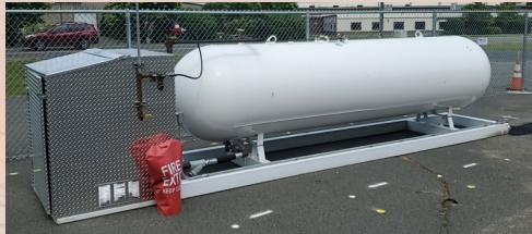
New Bulk Propane Tank Filling Station
